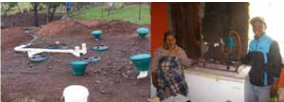
Biodigester installation with the outflow of digested cow dung (left) and a biogas stove at Maloka farm with desulphuriser to absorb odour, and a pressure gauge to measure biogas production (right).
